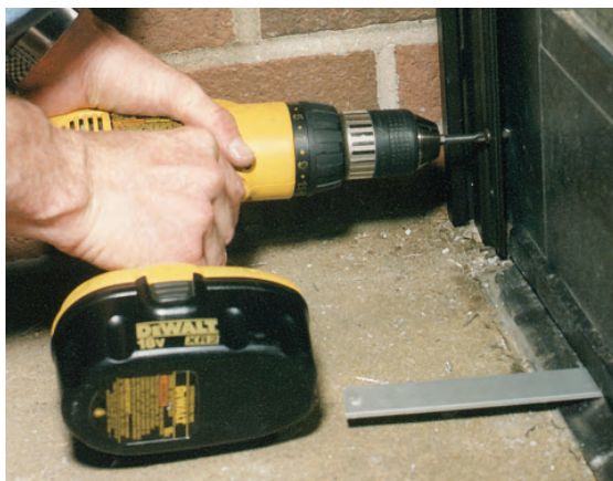
▲ Installing the bottom locator screw in the door leaf. Note the shim supporting the door, assuring proper threshold clearance.
