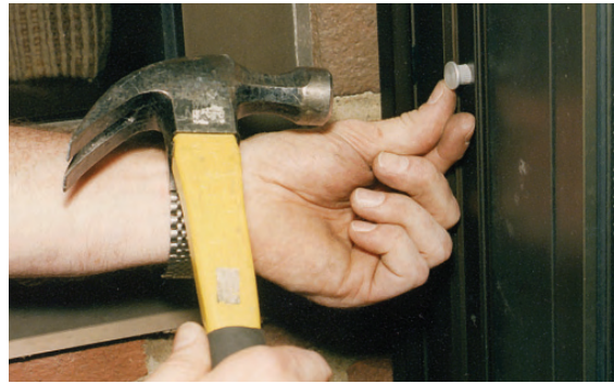
▲ Tapping in the barrel half of a through-bolt to secure the door leaf to the outside of the door.
